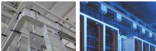
Containment & airflow racks
